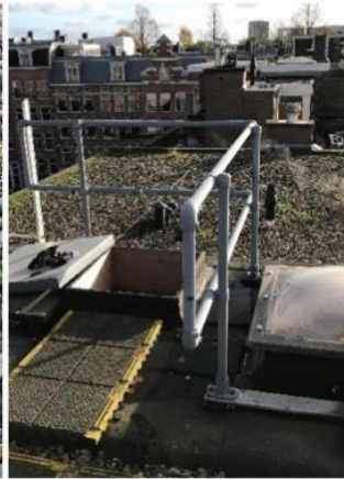
Entrance to the roof. iButtons have been placed on the ceiling of the hallway
