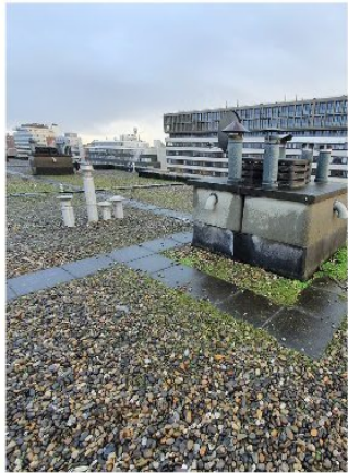
Roof surface of reference roof (gravel) at Oosterparkbuurt. iButtons have been placed at the northside of the chimneys
