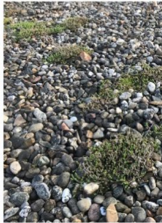
Substrate of blue-green roof at Oosterparkbuurt. iButtons have been buried under the substrate
