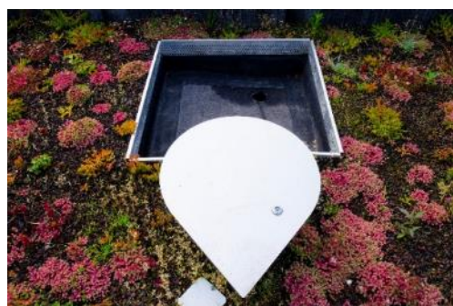
Figure 4 A smart valve as implemented on one of the RESILIO pilot roofs.
