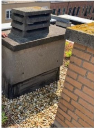
Roof surface of green roof at Oosterparkbuurt. iButtons have been placed at the northside of the chimney
