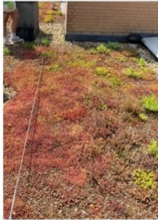
Substrate of green roof at Oosterparkbuurt. iButtons have been burried under the substrate
