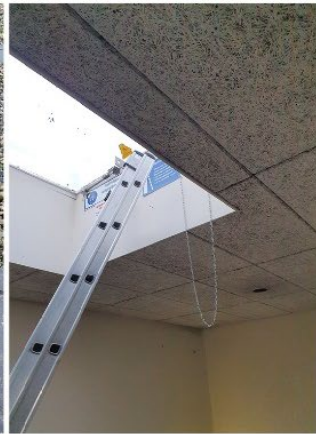
Entrance to the roof. iButtons have been placed on the ceiling of the hallway
