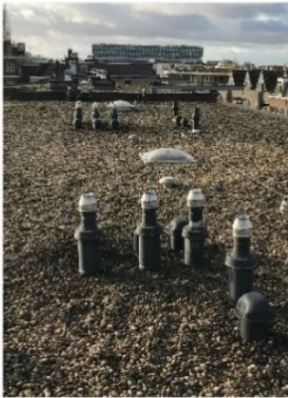
Roof surface of blue-green roof at Oosterparkbuurt. iButtons have been placed at the northside of the chimneys
