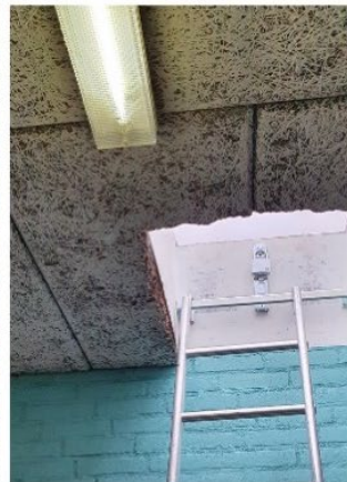
Entrance to the roof. iButtons have been placed on the ceiling of the hallway
