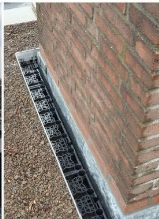
Example of the water crates installed under the substrate. iButtons have been placed in the crates
