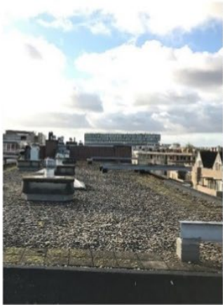
Roof surface of reference roof (gravel) at Oosterparkbuurt. iButtons have been placed at the northside of the chimneys
