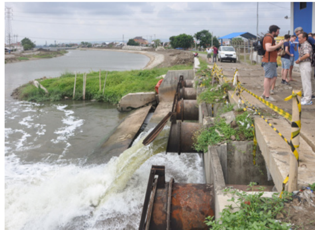
Pumping station in the Banger Polder.
